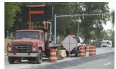
Henrico Department of Public Utilities plans to wrap-up construction on its latest Gaskins Road project by late September.
