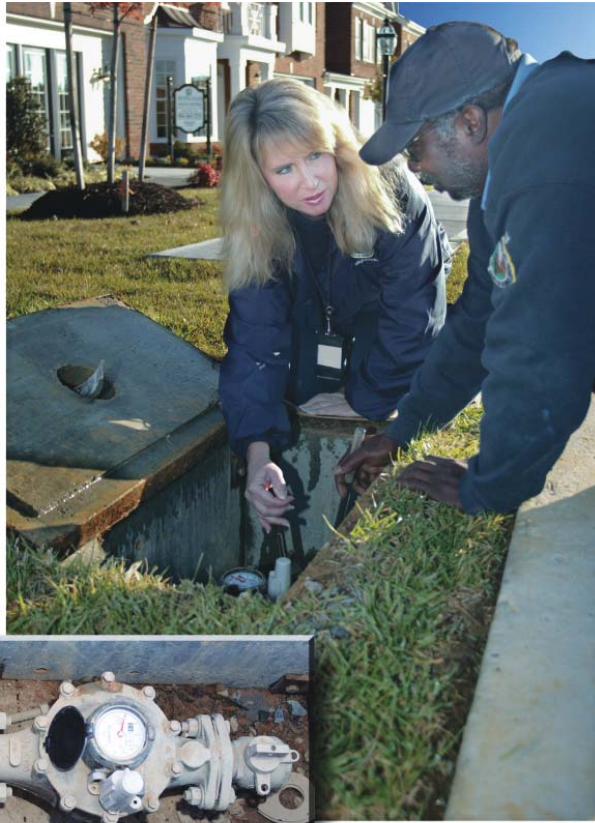
Public Utilities staff members Ivy Keck, left, and Randy White install a new Auto Read water meter in a Henrico neighborhood. The county is in the process of converting its 94,000 water customers to the automated meter reading system, which uses wireless technology to track water usage.
