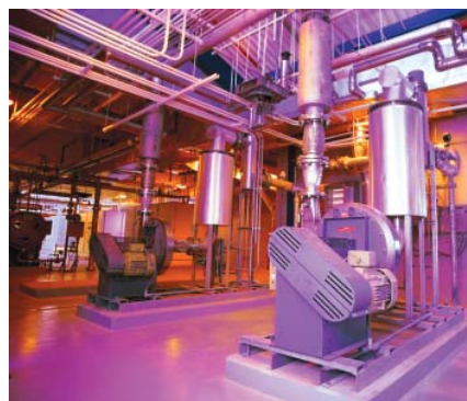
Henrico’s Water Treatment Facility was recognized for excellence in performance by the Virginia Department of Health’s Office of Drinking Water.
