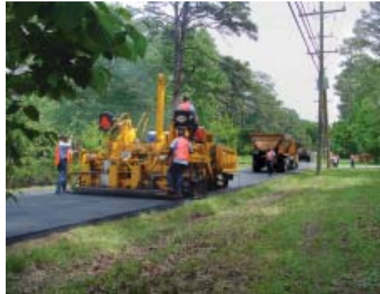
Henrico County is one of only two localities in Virginia to maintain its own roads. Shown here, a Public Works crew repaves a section of the county's 3,088 lane miles of roads.
