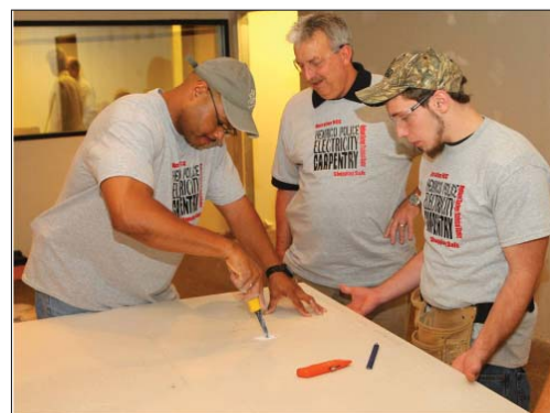
Henrico Police Capt. Eric D. Owens (left) cuts a hole in a piece of wallboard as part of work to open Central Station at Virginia Center Commons. Capt. J.C. Coover (center) looks on as Roger Culbertson, a junior studying carpentry at the Highland Springs Technical Center, steadies the board.
