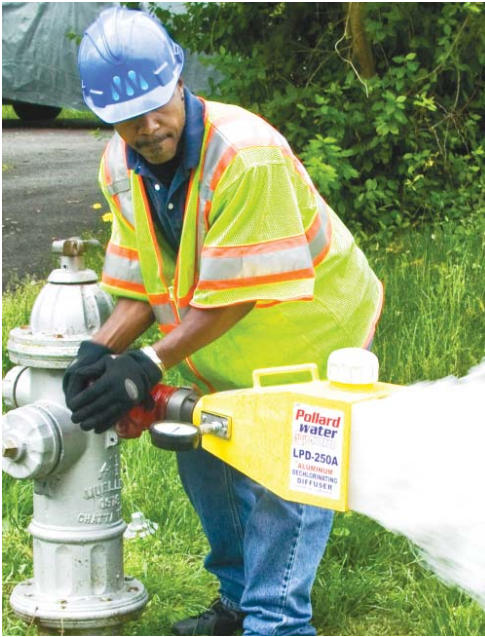
A 10-year program to clean Henrico's water mains is under way. Crews recently flushed this main near Nine Mile and Echo roads.
