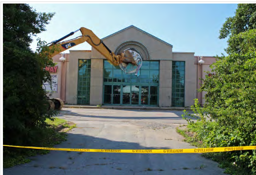
Demolition crews ceremoniously tear down the Fairfield Commons mall on Thursday. Photos by Katie Demeria.
